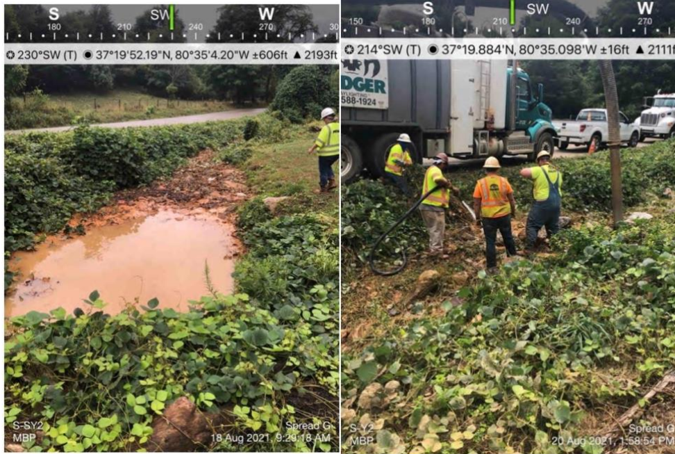
Figures 2 & 3 - MVP damage to Doe Creek and "mitigation" with pressure washers
