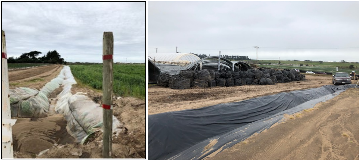
Figure 10: Plastic lined ditches control erosion but are vulnerable to breakage. Broken pieces can be transported to the ocean with storm water.
